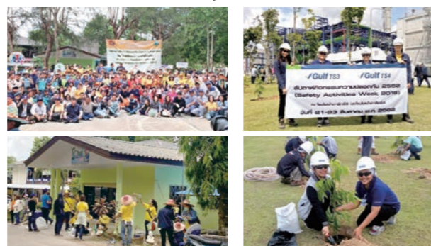
Upper left / lower left: Renovation and painting work at Ban Khao Wang Man School in Thailand
